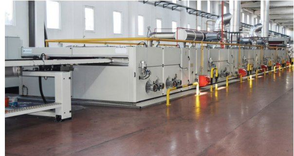
Fig. 13. A stenter machine with economizer installed
