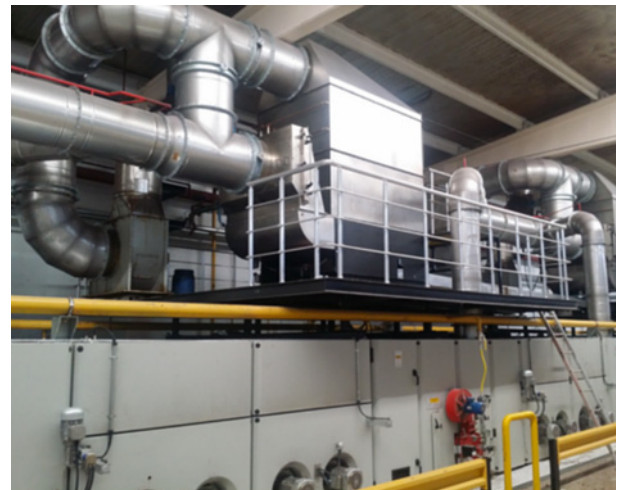
Fig. 14. Image of economizer on stenter machine
